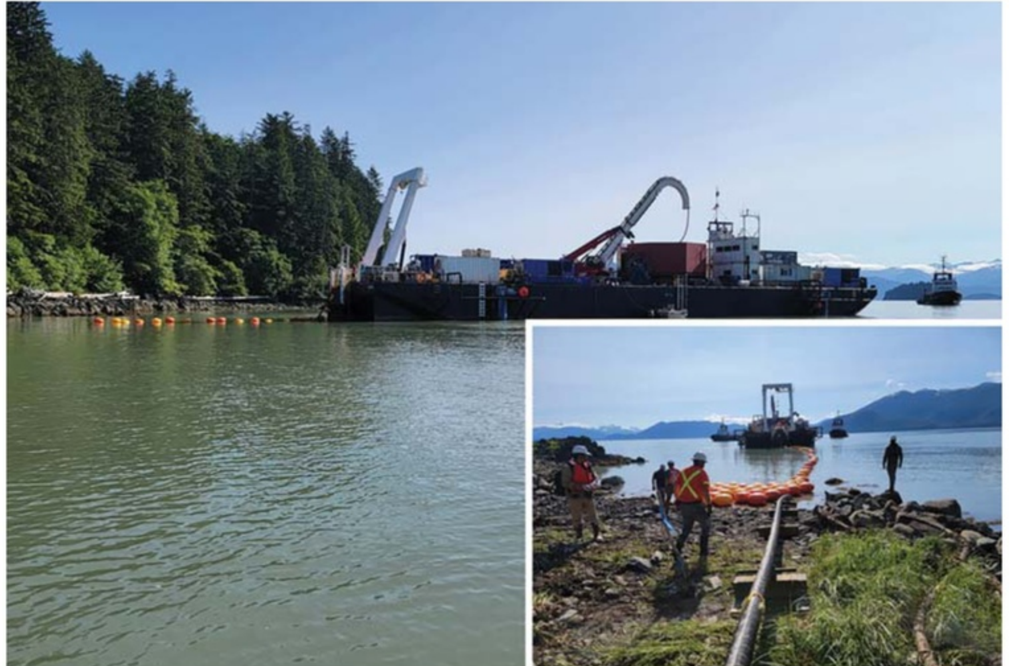
Installation of the 69 kV XLPE insulated cable, Vank Island, Alaska. Photos by SEAPA.
